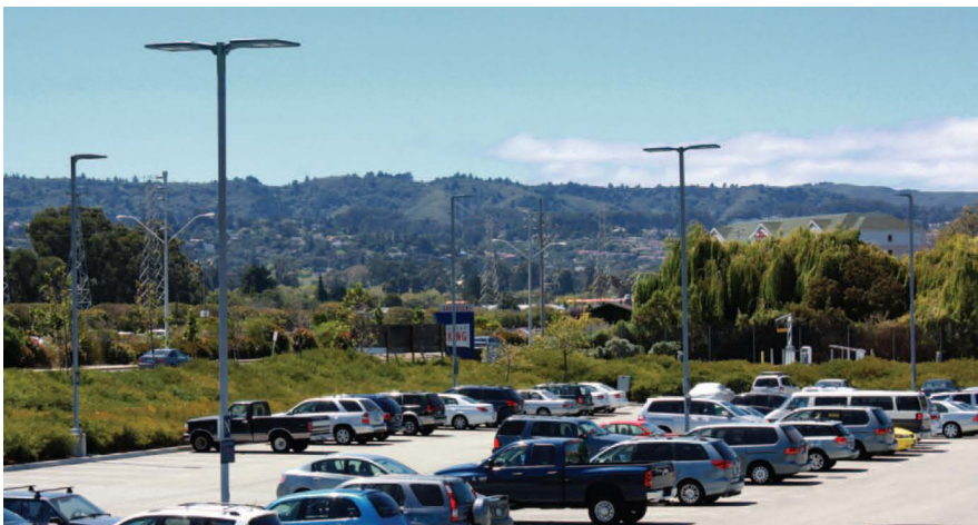
LED Parking Field Lighting Poles
